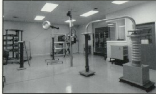
Above is shown the 70kV Hi-Pot/Partial Discharge - Corona Test Equipment
