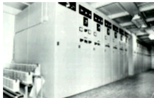
Interior Switchgear of Climatized Unit
