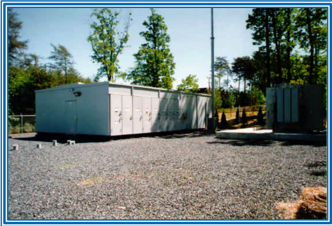
OUTDOOR, METAL-CLAD POWERCON SWITCHGEAR
