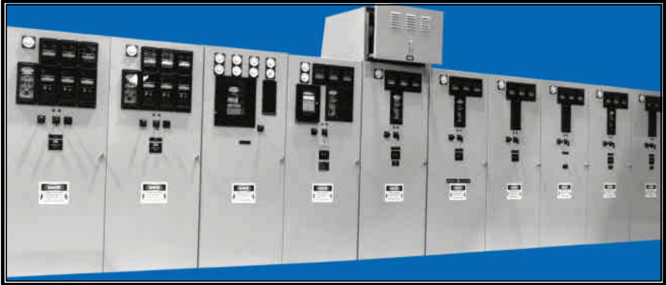
Typical 13,200 Volt Switchgear Rehabilitated to Better than New Condition
