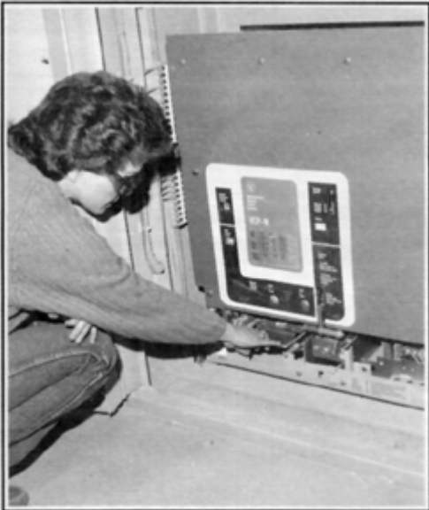
BREAKER IN TEST POSITION
