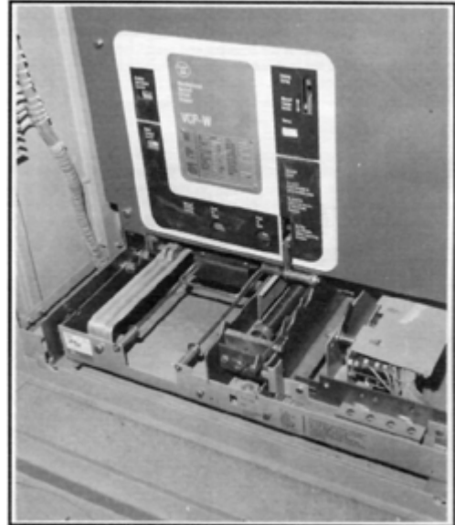
BREAKER RACKED INTO INTERMEDIATE POSITION
