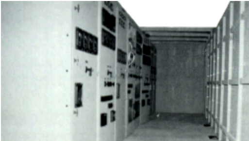
Outdoor Walk-in Metal-Clad During Final Assembly
